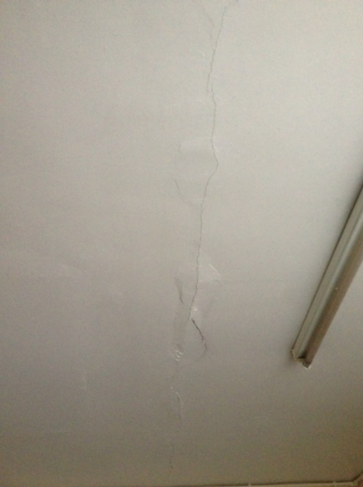
Office areas G224-232. Example of cracking to soffit with evidence of potential continuing movement.
