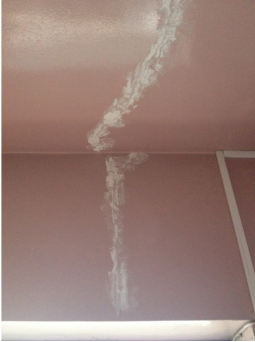
Office areas G224-232. Example of cracking to soffit with evidence of potential continuing movement.
