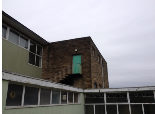
Elevation E10A, repairs recommended repairs not carried out. Loose stonework to corner needing repair.
