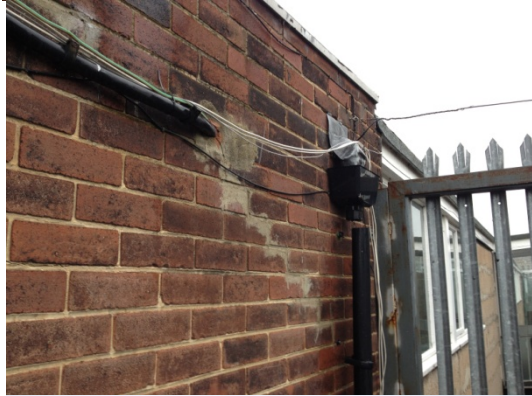
Cracking to NW end of roof 2, no elevation reference showing potential evidence of continuing movement.
