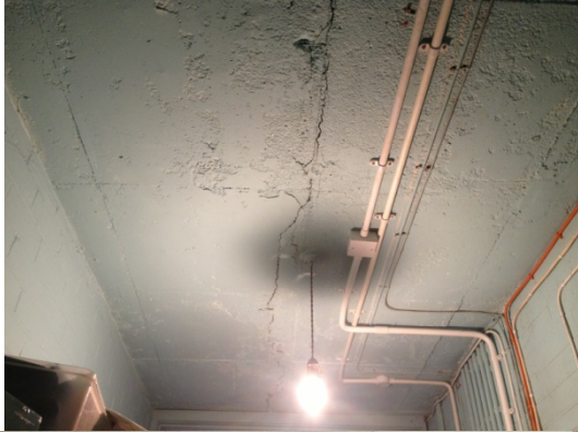
Office areas G224-232. Example of cracking to soffit with evidence of potential continuing movement.
