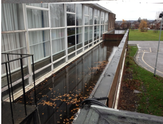
Significant ponding to flat roof area 3.
